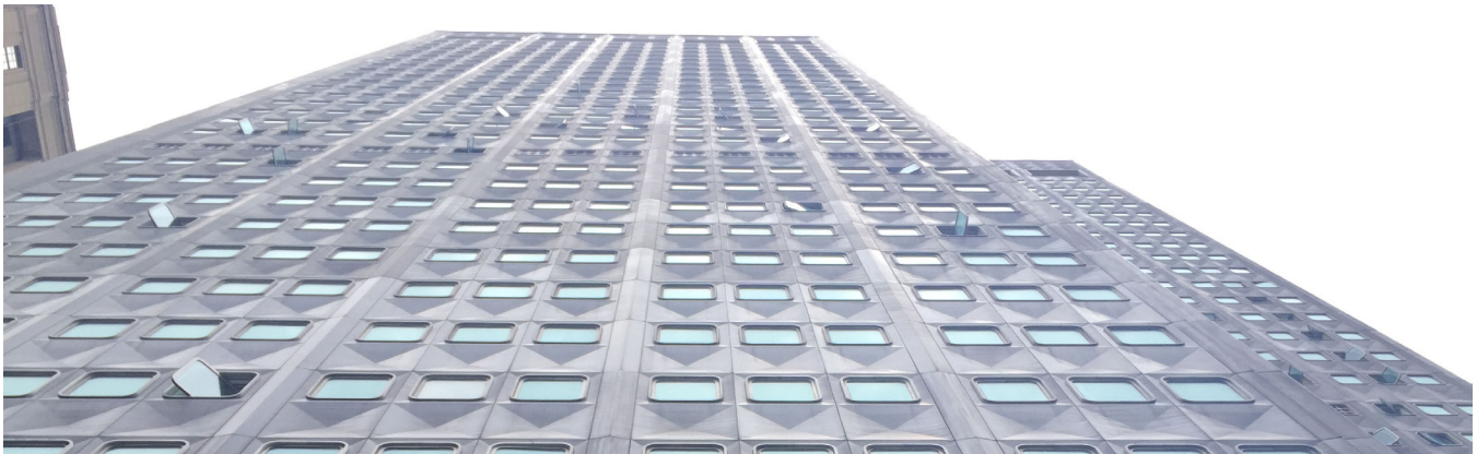
Figure 1. Aluminum cladding on the Alcoa Building (1953). Image Credit: Photograph by the author.
